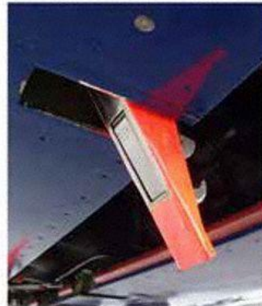
(e) Cowls open on hold open device, latch handle hook engaged. Cowling not locked.
